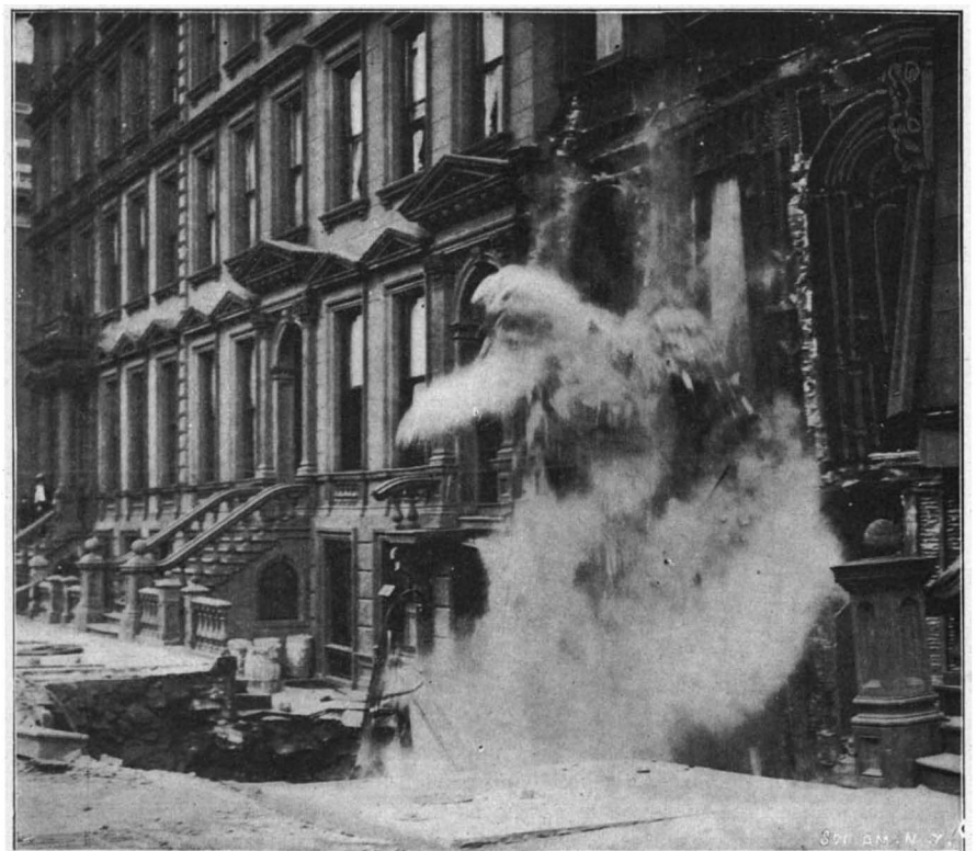
Snapshot Taken as the Front Walls Collapsed.
