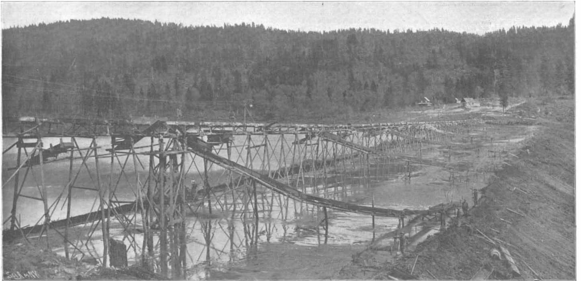
Where the Filling of the Dam Confining the Reservoir is Being Sluiced in.
