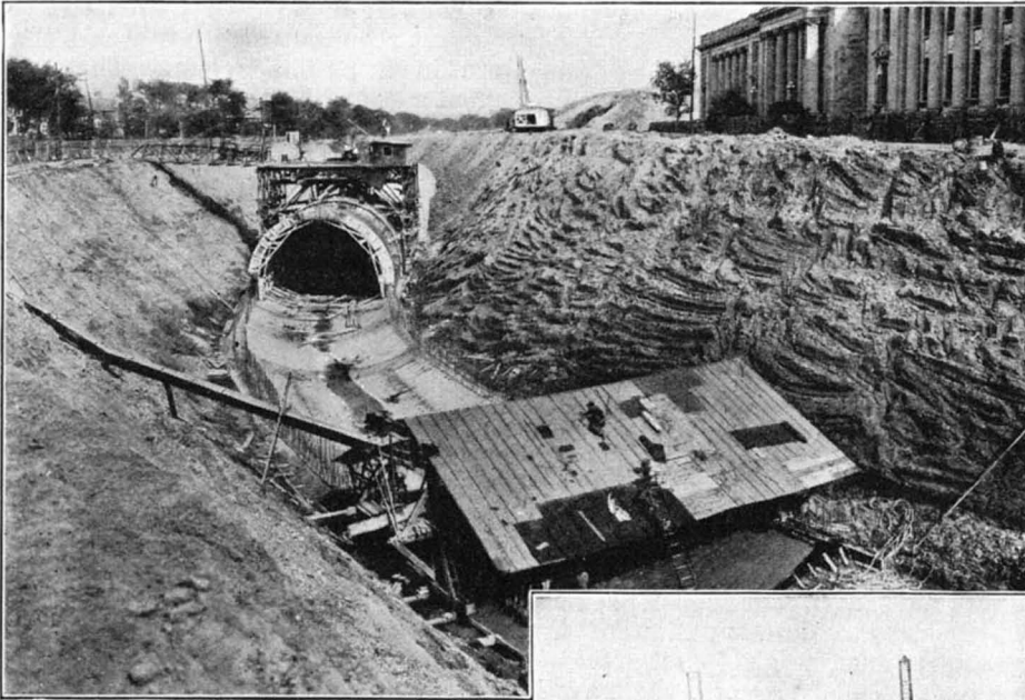
The single 32-foot sewer in process of construction in front of the Jefferson Memorial Building
