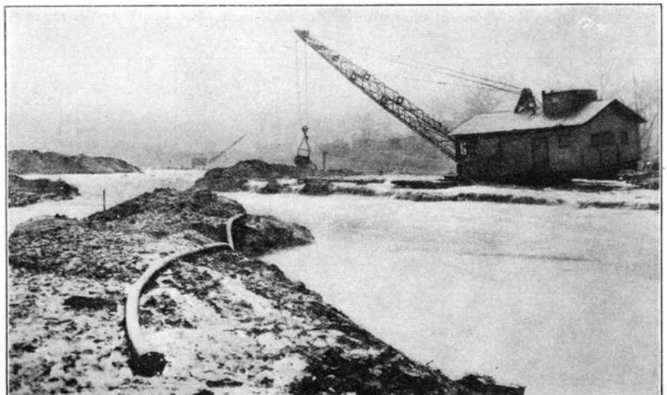
A section of the job showing one of the heavier floods passing over the construction work. The crests of these floods usually were of a few hours' duration
