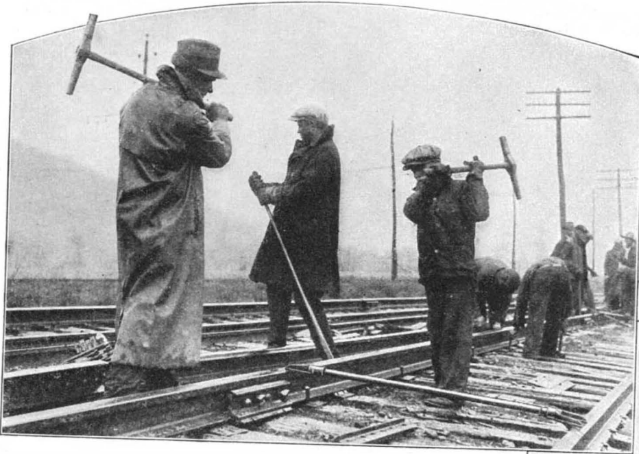
The new track is set in the proper position with the aid of a track gage and is being fastened to the ties by trackmen
