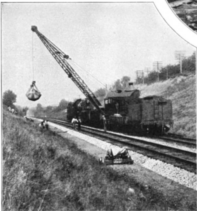
Shaping the hillside so as to intercept drainage from the tracks. A locomotive crane is used
