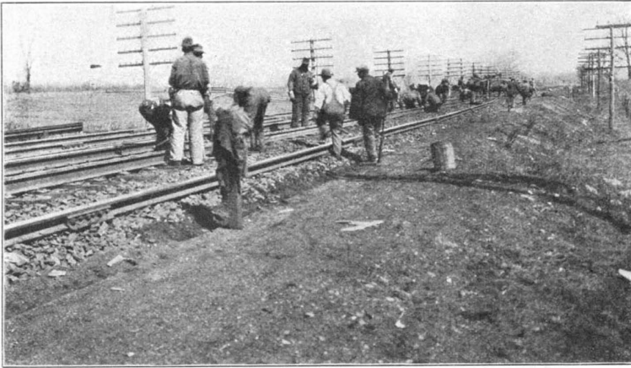
The new rail is placed as quickly as possible so as not to interfere with the movement of traffic and the old rail is slipped to one side and dismantled later
