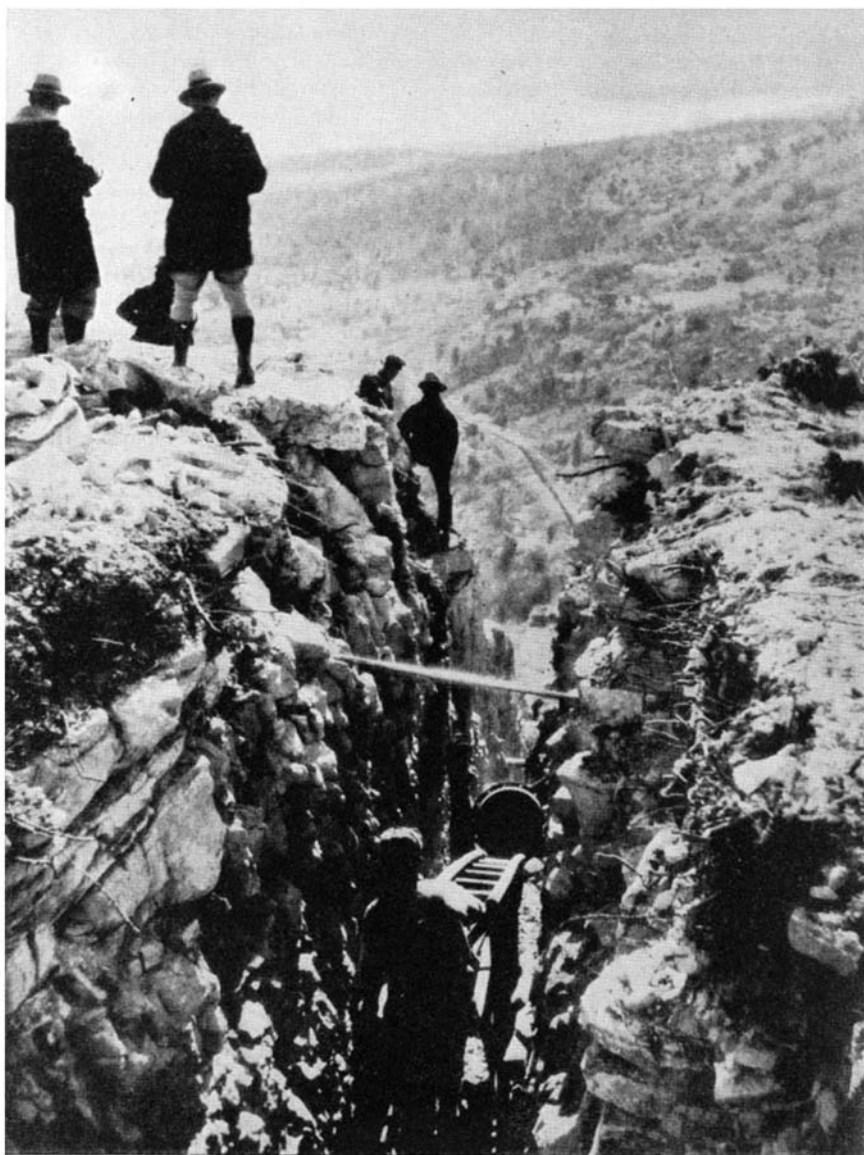
A rugged ten miles of scenery on the Denver gas line. In distributing gas from the fields, pipe-lines must be laid across mountains and through rivers
