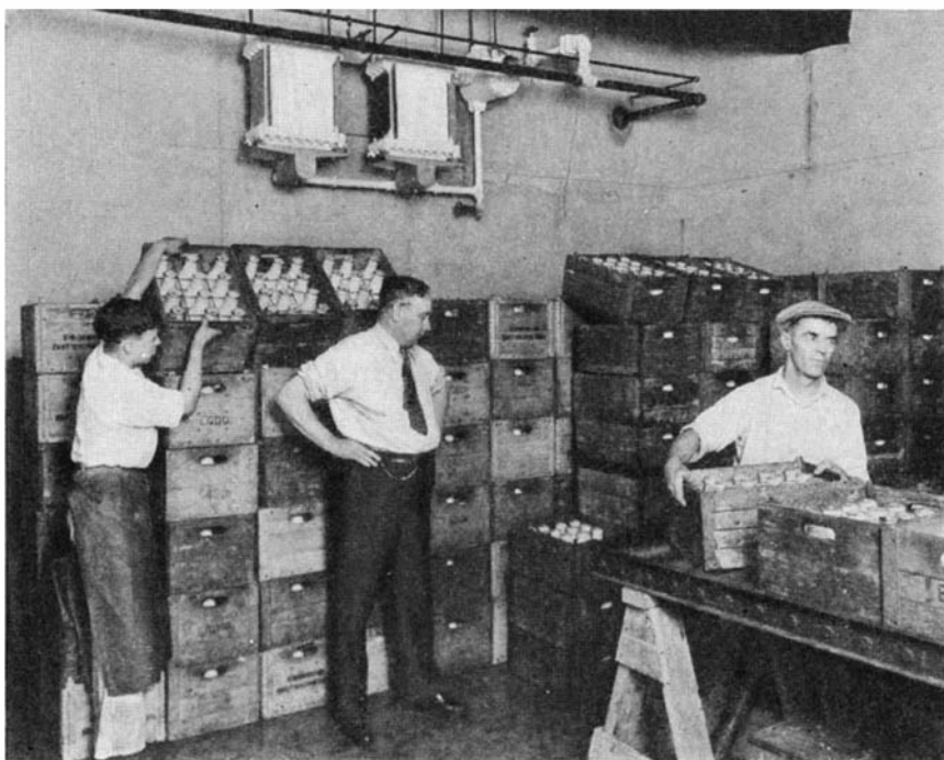
A refrigerated storage room which has no maze of pipes nor any drip of condensed moisture. The automatic refrigerating unit is shown on the wall at left
