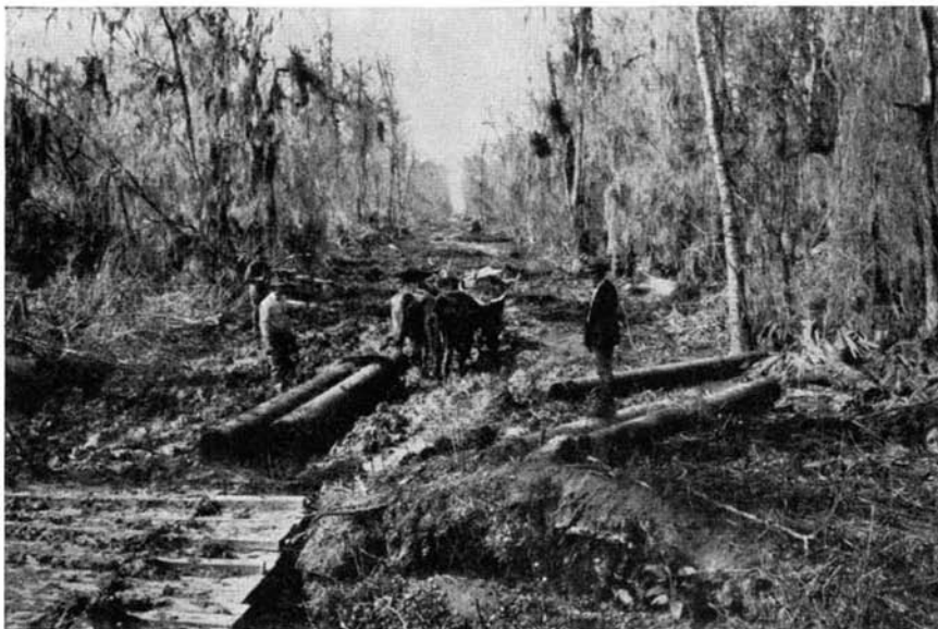
Back to the primitive. In swampy land such as this, oxen and mules have proved to be about the best motive power for transporting pipes for the pipe lines
