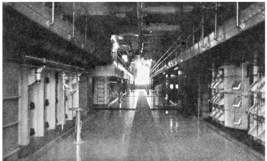
White uniformed "stokers" work in this "ball room" which is, in reality, a furnace and boiler room. The popular idea is that this is a place of ashes and coal
