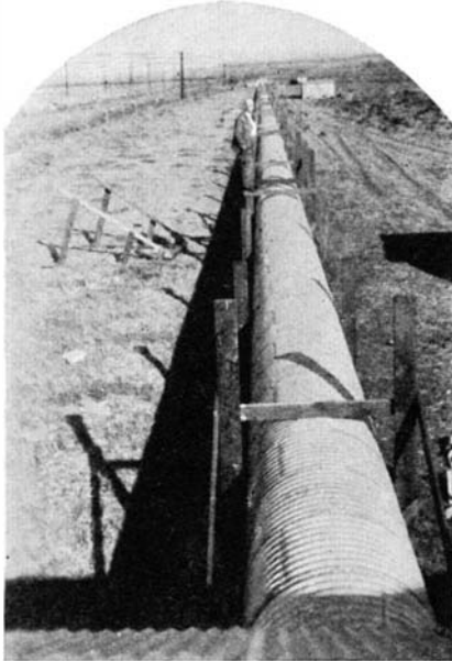
The long vacuum pipe is about 35 miles to the southeast of Los Angeles
