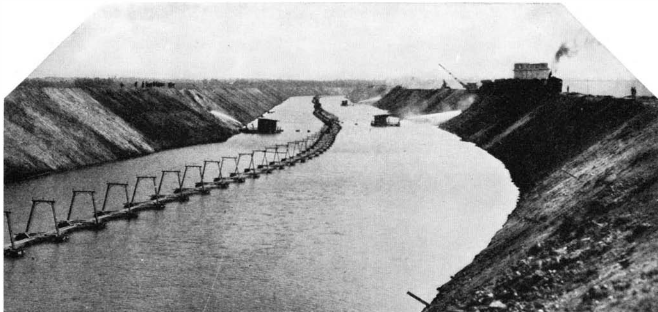
The segregation pool in the core trench of the dam. Trains dumped their loads of earth down the side banks; and powerful pumps on several scows shot streams of water on this loose material, washed it down, and settled it firmly
