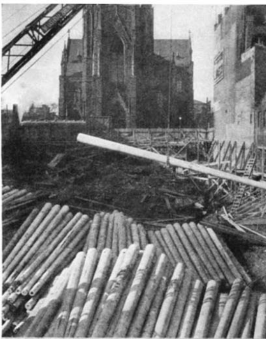
One of the new piles is lifted from the supply at the site of a new building in Buffalo, N. Y.
