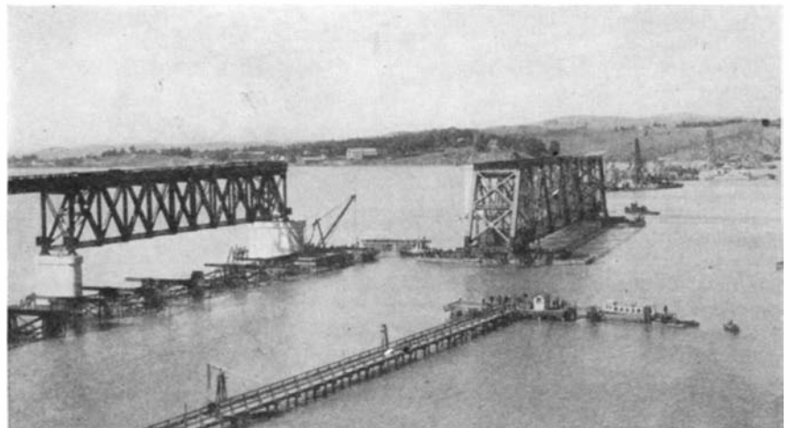
Deck span being floated into position between piers. It served as falsework for construction of the permanent through truss spans between each pair of piers
