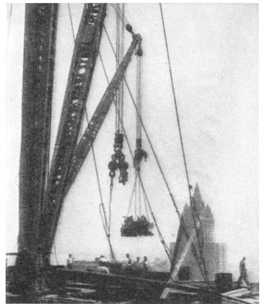
Giant derricks lift part of the hoisting machinery to be used by the constructors
