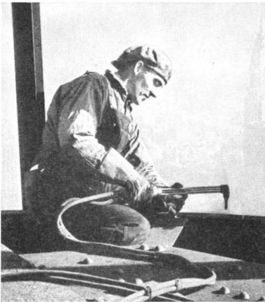
Oxy-acetylene torch used to cut notches in beams for inserting concrete floor reinforcing
