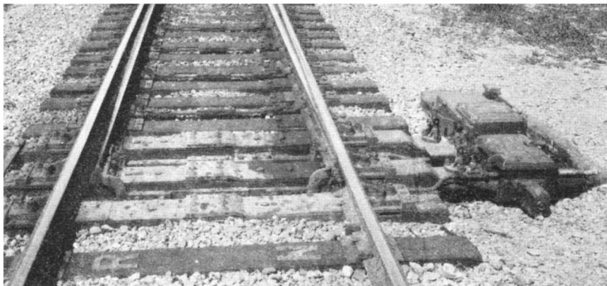
Dual-control switch leading from the main line to a siding, and the switch mechanism which is operated by electric motor or, when necessary, by hand
