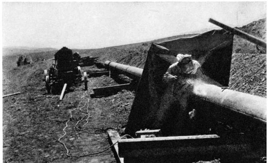
Extensive pipe-line systems for natural gas and oil have been made possible by the perfection of new processes for welding the joints between pipe sections
