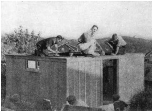
Figure 5: The circular track was permanently attached to the top of the wooden structure
