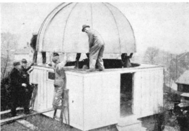
Figure 10: All hands picked up the dome, walked it aboard the building, and tenderly lowered it to position
