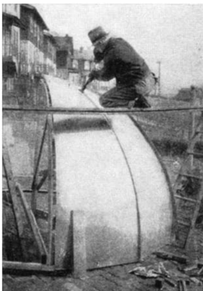
Figure 7: The iron polygon shown in Figure 6 was dismantled and the gores were attached one by one
