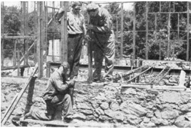
Building the two-story, six-room dwelling of arc-welded steel frame-work. A frame panel being welded to a sill
