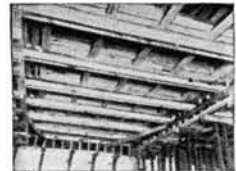
With the Presdwood forms, there was a reduction in size and quantity of lumber used. Shoring was used under beams only; no re-shoring required. Quick erection and stripping helped to reduce cost
