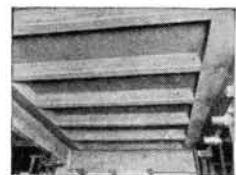
Note the smooth surface of the concrete—no grinding, extra finishing or plastering required. After being stripped, the Presdwood used was removed and made into forms for other concrete construction
