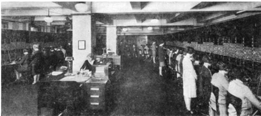
A private branch exchange which takes care of 1600 stations. Through it incoming calls are distributed and various extensions may call each other
