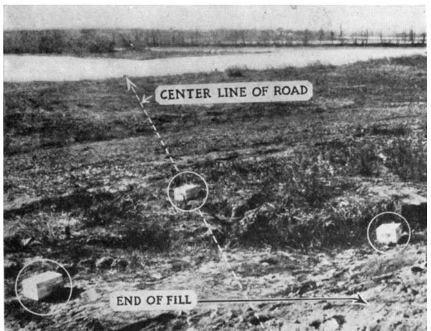
Boxes of dynamite arranged on a "three point" system of loading, before depositing fill material on right of way. See bottom diagram on opposite page
