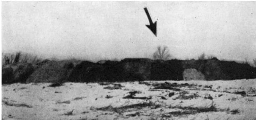
Fill material piled within road lines before sub-surface blasting. For either three-point or casing loading the material should be piled high for a deep fill
