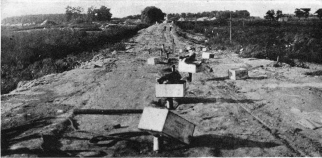
Casings in place in a highway fill, ready for lowering of dynamite
