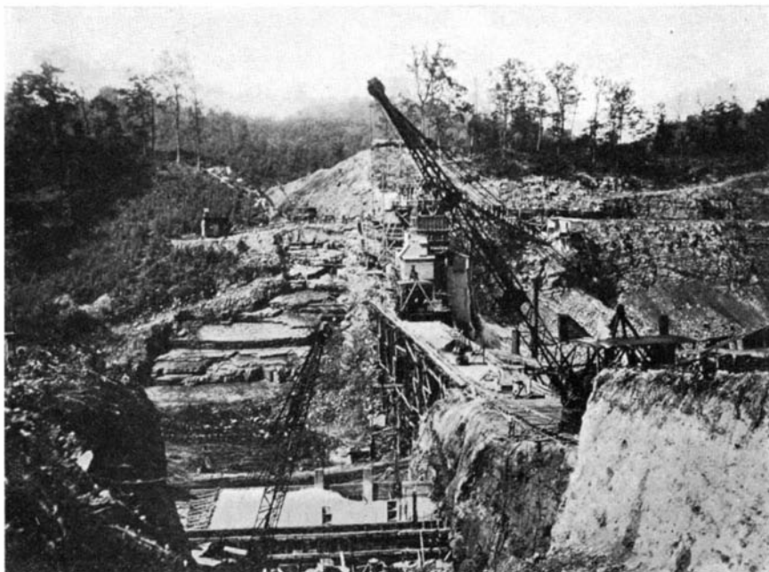
Stripping operations on the site of the Koon Dam in Pennsylvania. To get perfect concrete, all materials going into the dam will be automatically weighed
