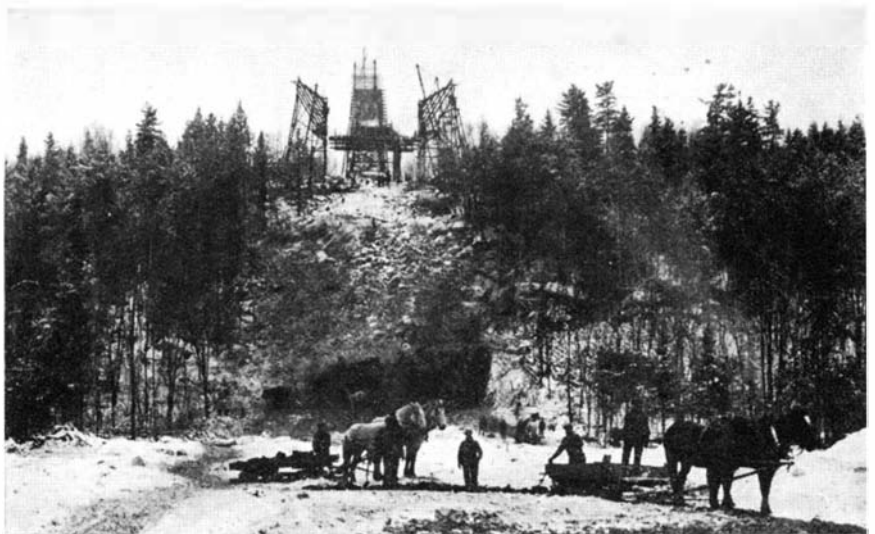
A view of the construction work on the jump. While the landing slope was being graded below the hill, the steel towers and the stands were erected above
