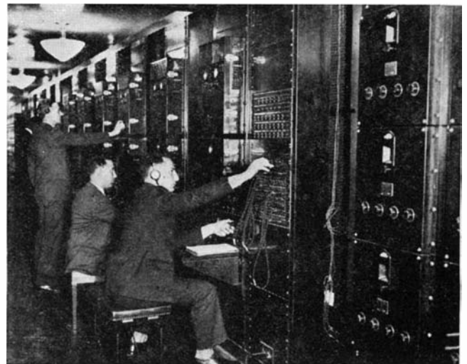
The control room of the Western Electric radio program distribution system installed for guests at the new hotel
