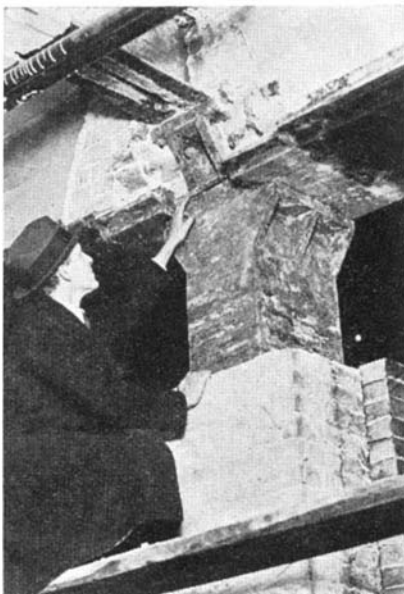
Further proof that the walls were supported by the columns alone
