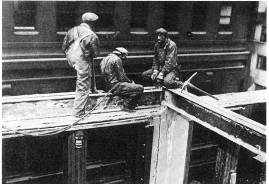
Removing the spandrel I beams at the fifth floor level. Uncovered details such as this were examined daily by the committee which studied the work
