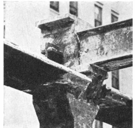
Method of supporting steel beams on a cast-iron column in an exterior wall of the demolished building
