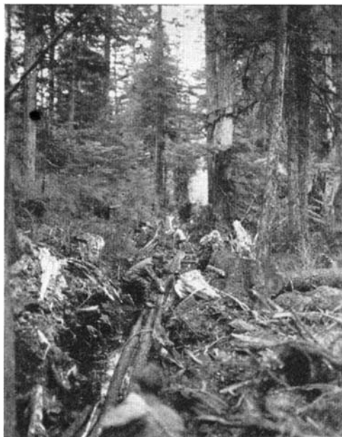
Laying a submarine cable over land. The spruce logs show the location of the trench
