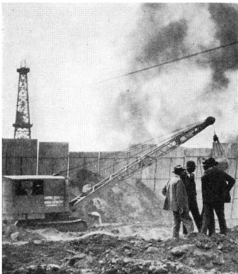
A shovel starts the excavation for a tunnel from which a gasser will be shut off
