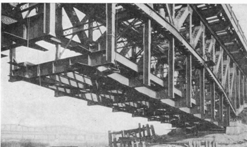
Construction of one of the ramps that are being built into the structure to permit its use by local traffic of nearby districts without interfering with through traffic
