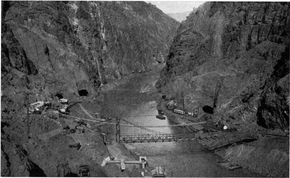
Looking upstream in Black Canyon. Downstream portals of tunnels 1, 2, and 4 are visible while that of tunnel 3 is hidden by the point at left of tunnel 4. Intake works of Boulder City water supply in foreground
