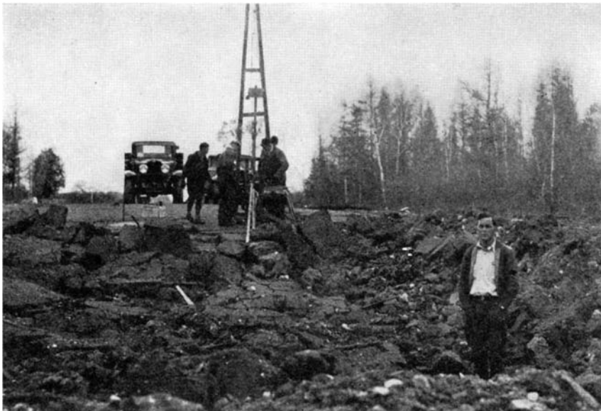
Extraordinary results of a blast to settle a highway fill across a marsh
