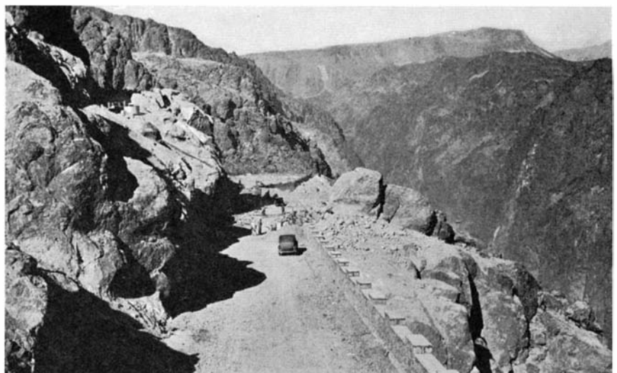
Difficult road construction work in a cliffside: Looking upstream along Black Canyon highway, with retaining wall and lookout point beyond point of rocks
