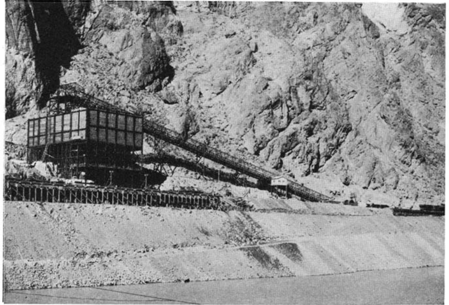
The great concrete mixing plant on the Nevada side of the river at the Boulder Canyon Project. Here concrete for lining the immense tunnels is being mixed
