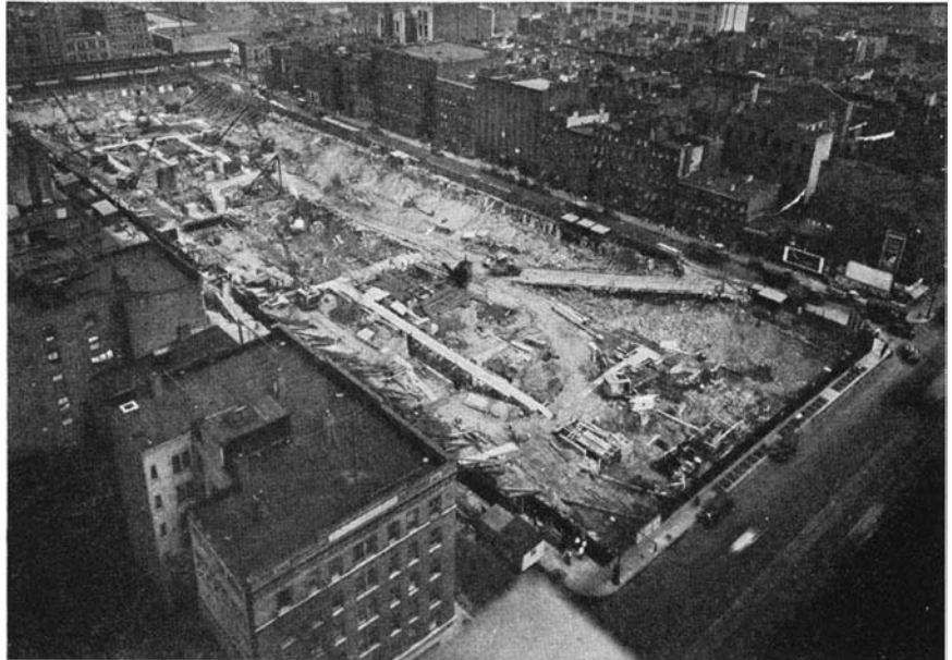
The great excavation necessary for the first of the three terminals, as it appeared in July, 1931. This gives an idea of the magnitude of the building
