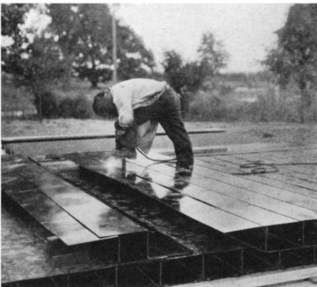
Assembling the floors on the foundation. When welded together, these "Z" sheets form a series of metal boxes
