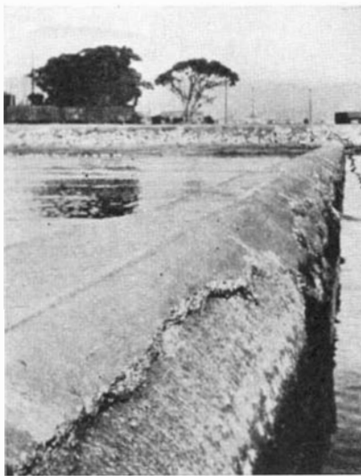
The exterior of a large concrete trunk sewer showing disintegration
