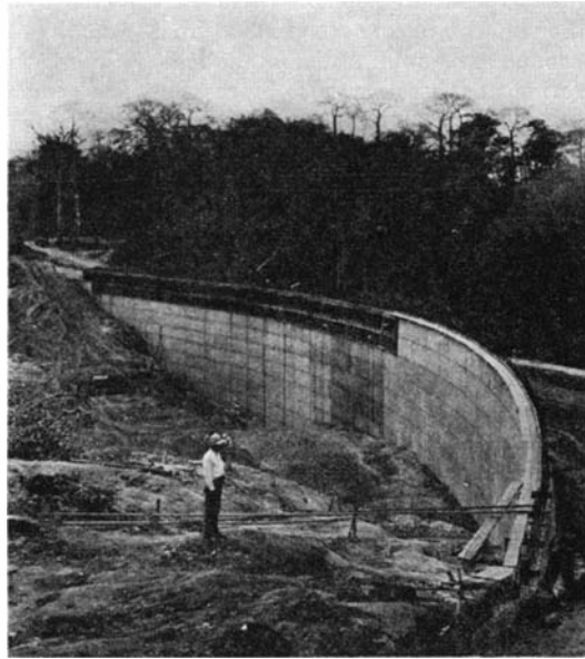
Concrete cut-off wall of one of the larger earth dams. Completed, this will be 58 feet high
