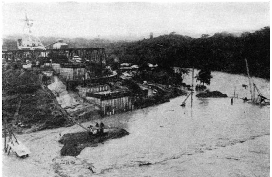
Looking southwest across the left abutment of Madden Dam during a flood of some months ago. Note the heavy machinery covered by this 112,000 c.f.s. flood
