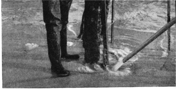
As a water jet displaced the sand the dynamite charge on a lath submerged to the required depth against the pile that is to be cut
