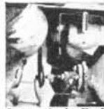
In every Statler Hotel, hot water is constantly kept at a safe temperature by automatic control, inspected regularly by an Engineer, as shown above.
