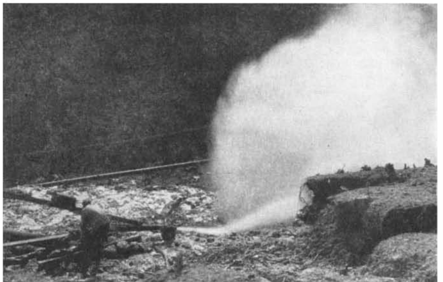
A view of the three-inch nozzle used in sluicing off the overburden on a quarry at the site of Norris Dam on the Clinch River, Tennessee. Water was used at a pressure of 100 pounds, and the overburden was washed off (Continued at right)
