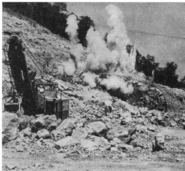
Quarry on the hillside above the dam site just as a blast was set off to produce broken stone for primary crusher
