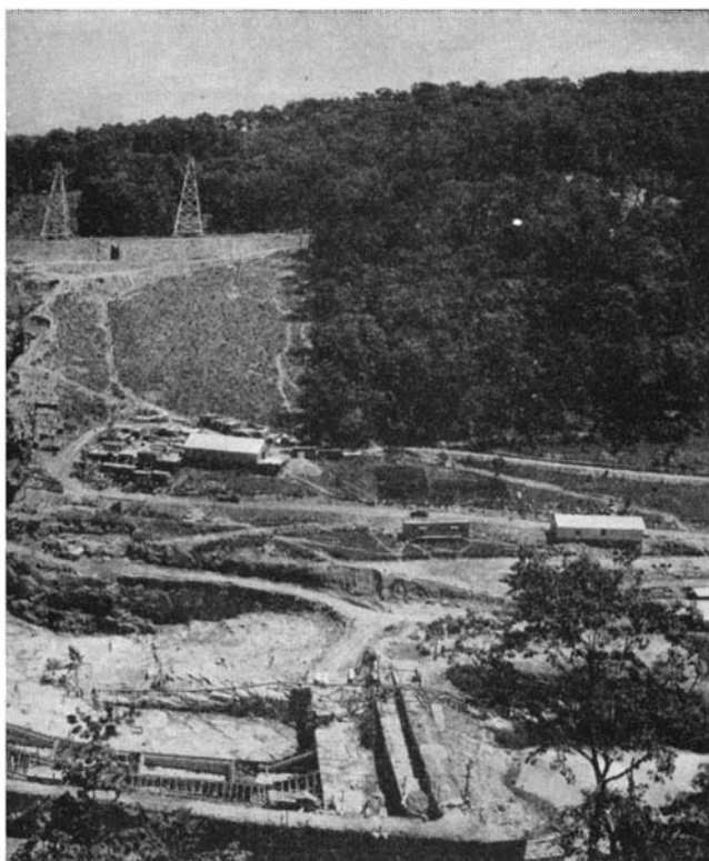
Norris Dam on the Clinch River shortly after pouring of concrete had been started in east coffer dam
