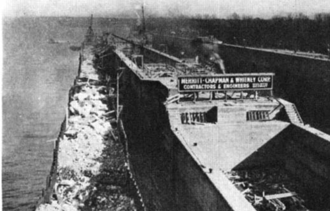
Early construction stages of Lock Number 15 (right) at Rock Island, Illinois. Rock-filled cofferdam may be seen at the left
