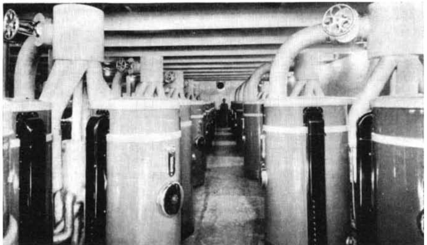
A battery of oil burners in a central heating plant
