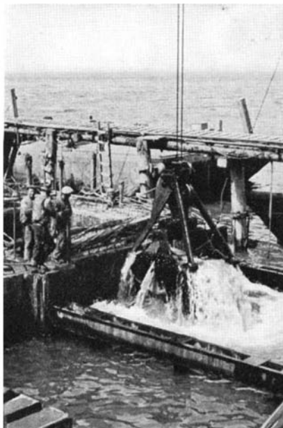
Final cleaning operations on one of the caissons. Clam-shell buckets replaced "sand-hogs" on this job
