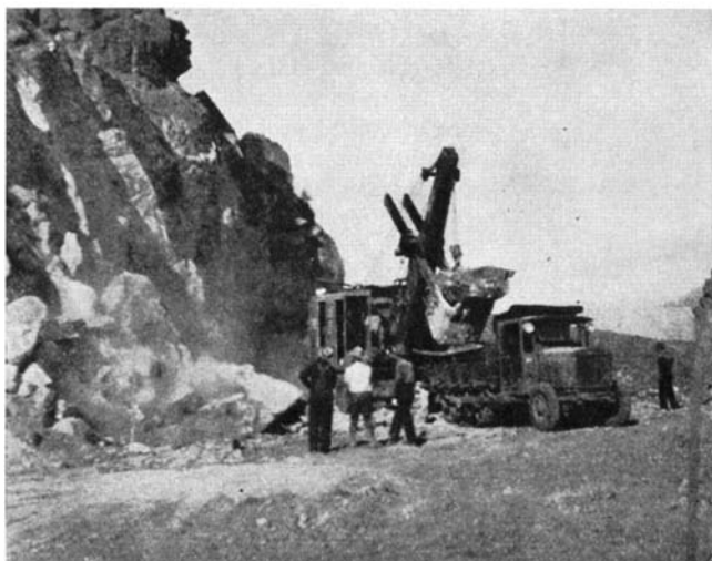
A truck and steam shovel moving huge granite blocks to clear the way for the railroad grade to the damsite
