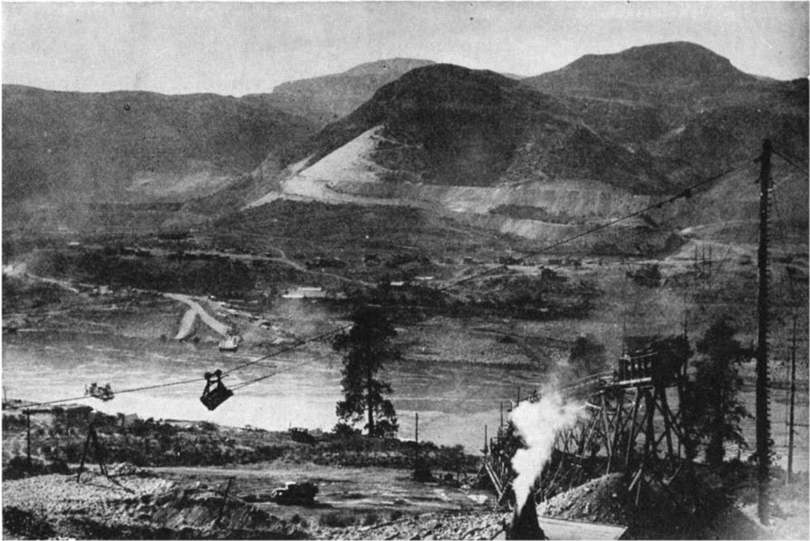
A view taken from the east bank of the Columbia River at the site of Grand Coulee Dam. Gravel washing equipment is in the foreground; across the river are the contractor's camp and Government road grades
