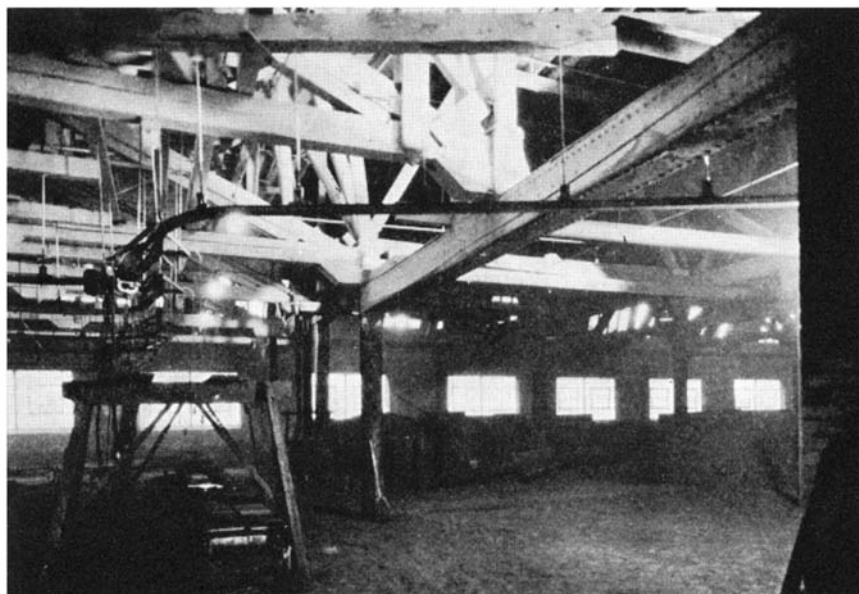
One of the surest ways to reduce efficiency in manufacturing processes and decrease worker morale is to delay repainting as was done in the plant shown
