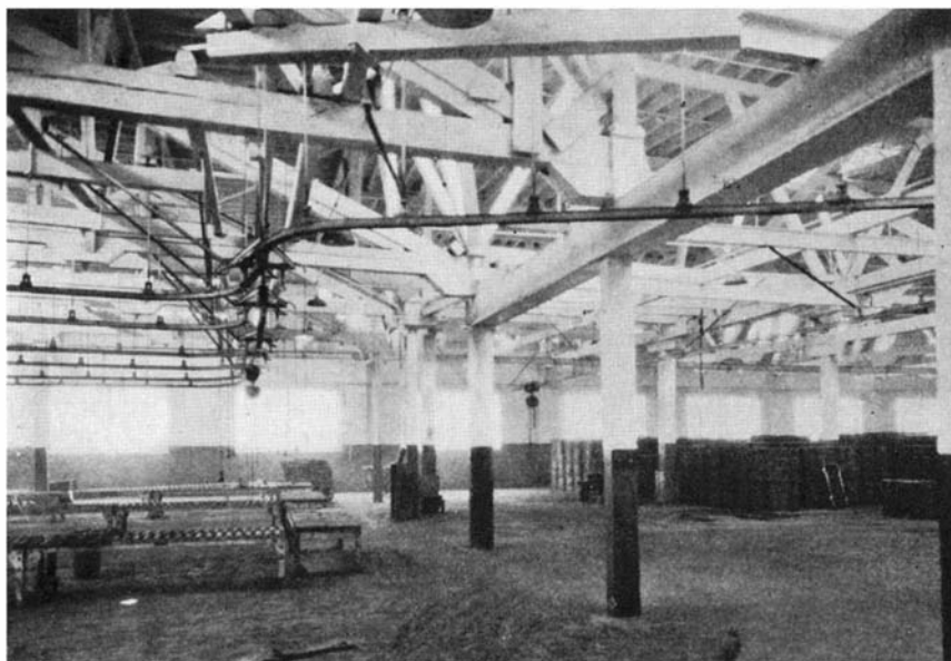
Under approximately the same lighting conditions as in the picture at left, the new paint job here pays dividends and promotes safety and worker contentment
