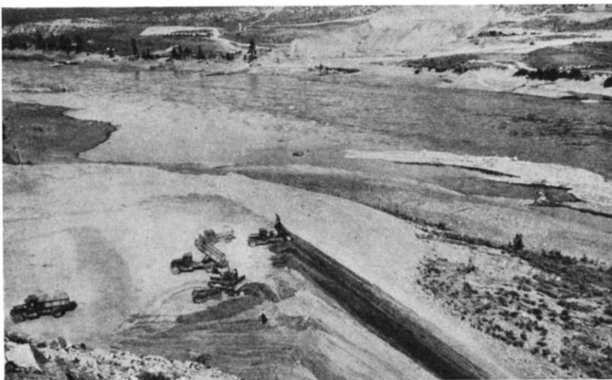
A spoil bank piled up by preliminary excavations at the site of Grand Coulee Dam. This bank forced up the islands visible at the right, and may have to be removed as work progresses and further excavations are made to reach bed rock
