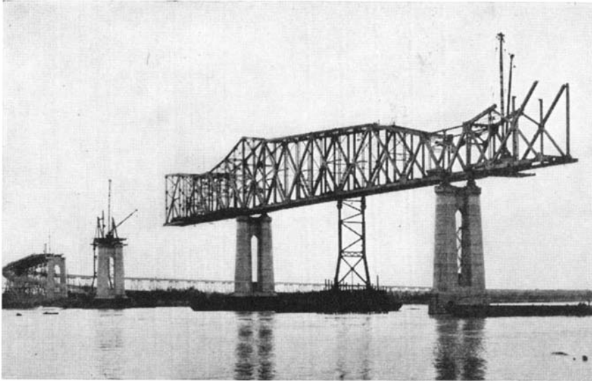
Erecting steel for the superstructure of the main bridge. The quick incline down from extreme left is the roadway; the gradual incline is the railroad
