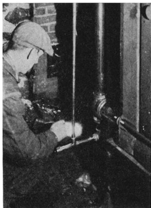
Sweating the fittings together in the newer type of copper alloy residential plumbing
