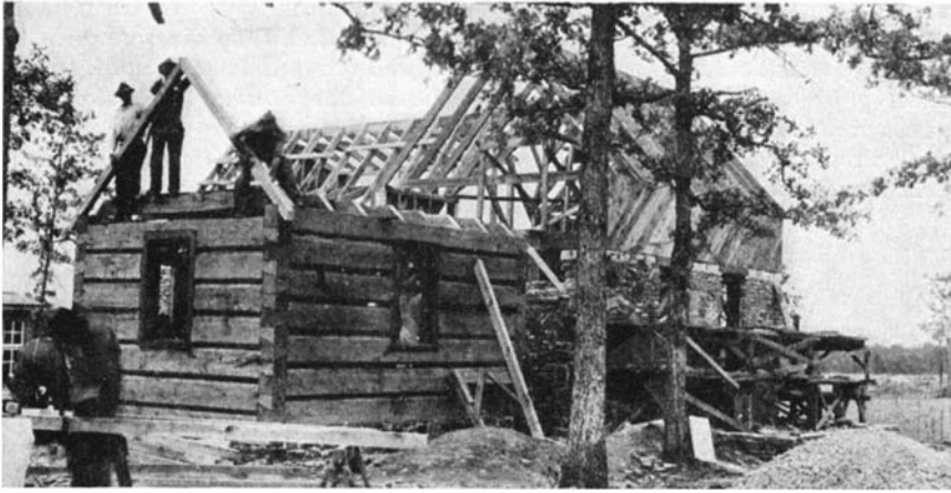
An attempt is made to uphold the traditions of the locality of each project. Here, under construction, is shown a modified log and stone house in Tennessee
