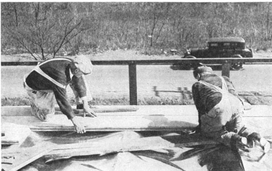
Laying the gypsum section of one type of "package" home. Long used as a heat insulator in steam plants, gypsum may find wide use in house construction
