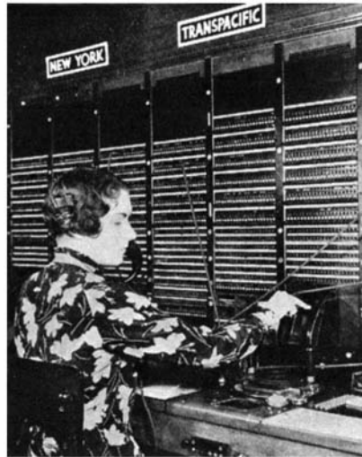
"Scrambled" speech is used in commercial radio channels to prevent eavesdropping. Transpacific calls go through this switchboard
