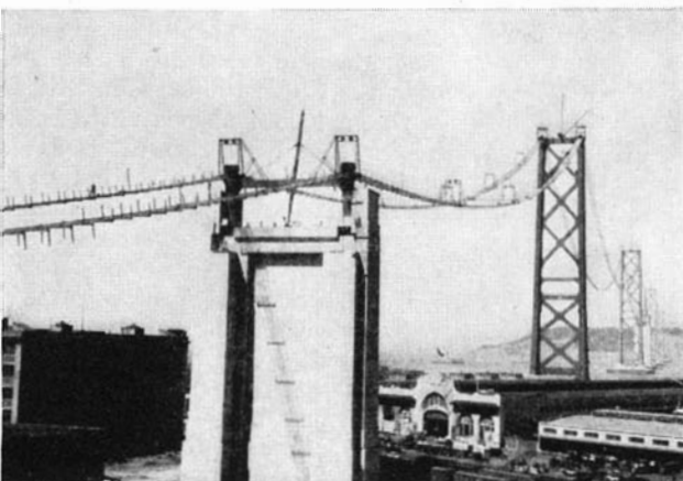
Below: A general view of the construction work, after the catwalks were completed and before spinning. Note the "gallows frames" provided to support the wheel cables
