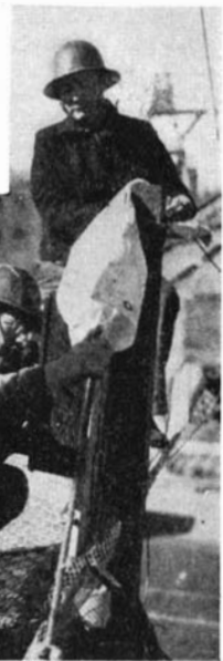
Left: A close-up view of strand shoes in place, ready for the beginning of the spinning operation. Shoes are fastened to steel girders firmly embedded in concrete
