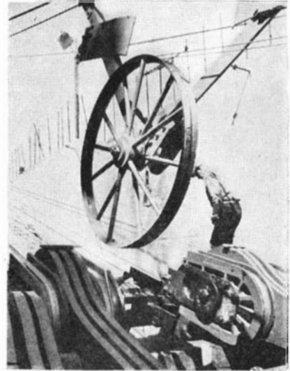
Right: The wires over the strand shoes near the edge of this illustration have been tightened to the correct tension. Above them is the wheel ready with two loops of wire for the return trip to the anchorage
