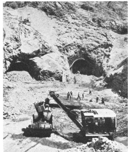
Ends of the two 29-foot horse-shoe type diversion tunnels built at Parker Dam
