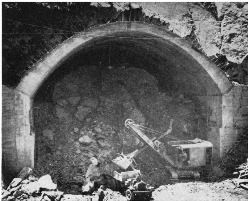
Taking out the core of the Yerba Buena tunnel, after the lining is in place
