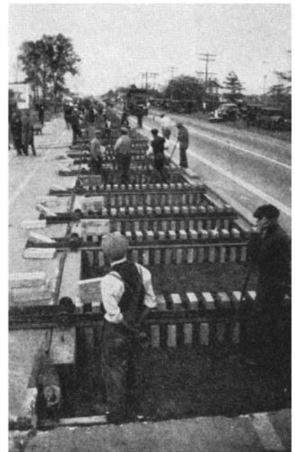
The highway strips are moved three inches at a time. Blocks are then inserted for the next sidewise "push"
