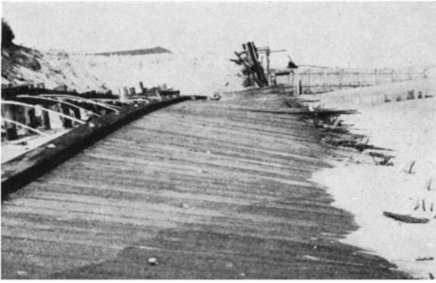
A timber bulkhead at Deal Beach that failed because the structure was not supported by a suitable back-filling
