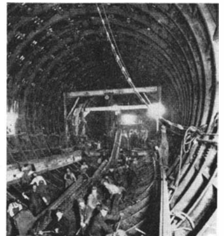
Placing steel work in one of the tunnels before lining with concrete
