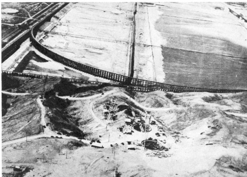
Looking westward toward the trestle-enclosed area. Dump cars used this trestle for placing the dam's gravel toes. In foreground are excavations for the valve shafts
