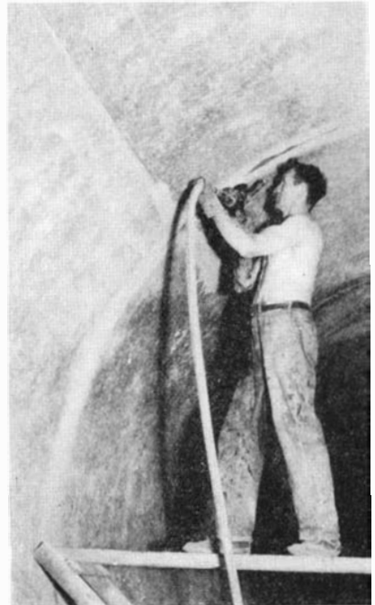
Smoothing the inner surface of one of the conduits with an emery wheel to reduce resistance to water flow
