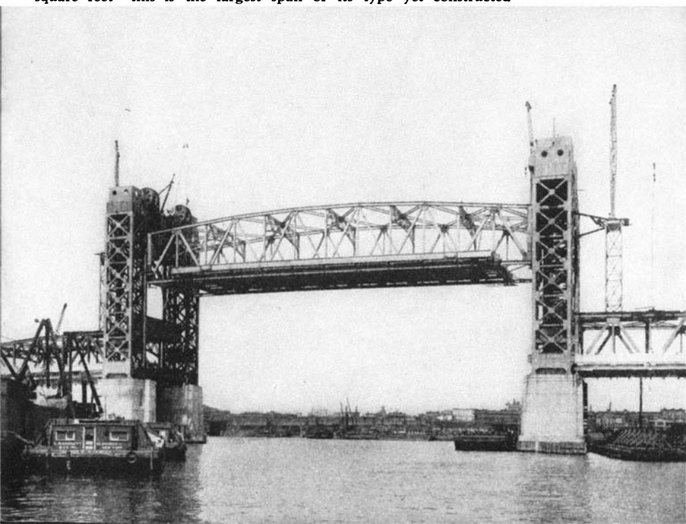
Vertical lift span in the Manhattan branch, during construction. The lift span has a length over the channel of 310 feet, is 55 feet above the water in lowered position, and can be raised to provide a clearance of 135 feet. Measured in terms of deck area—29,000 square feet—this is the largest span of its type yet constructed
