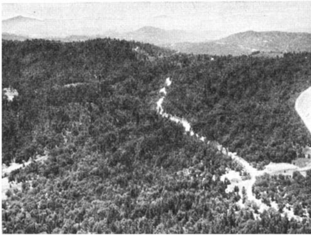
Scenery surrounding Mt. Palomar, where the great new observatory is being built. View looking in a southerly direction, showing the road which is being constructed up to the plateau—which is at 6125 feet above sea level
