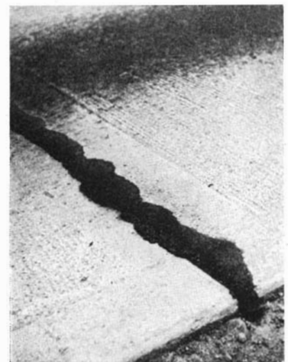
Solid asphalt expansion joint filler mushroomed out; result—a bump
