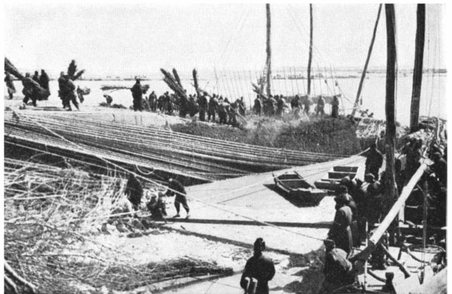
Pushing north end of the closure work into deep water. Note numerous ropes
