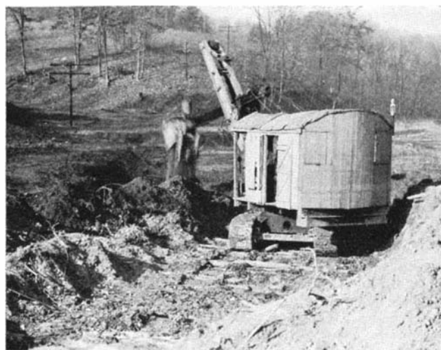
A steam-shovel stripping off the overburden preparatory to the digging of a deep trench, later to be filled with dirt
