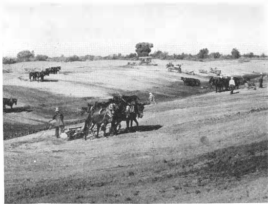
In some sections, it was possible to do the necessary excavating for the canal with mule-drawn scoops. However, three tractors are shown assisting at this spot
