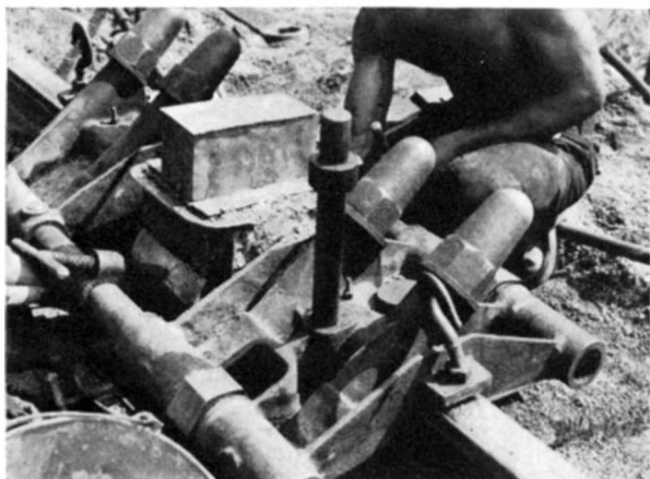
10 Long lengths of welded rail, in position, are joined by Thermit "closure" welds. Heavy clamps hold the rail in alignment while molten metal is poured into the mold. It requires about one hour to make a Thermit closure weld
