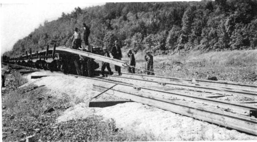
Unloading lengths of welded rails for distribution alongside of a track that they will eventually replace. A cable fastened to the end of one of the rails is anchored to the ground and the train is hauled away. The rail thus practically "unloads itself"
