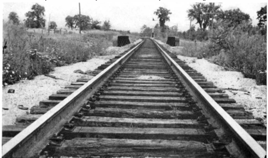
11 Welded rail in a finished track. Note absence of plates used to join conventional rails. Welded rails are laid in long lengths, broken only at intervals by the insulated joints necessitated by the usual signal circuits
