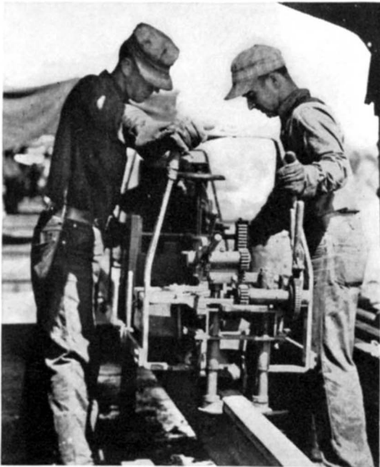
6 The fourth and final grinding. An accurately controlled abrasive block smooths and contours the rail. Welded joints eliminate the "click" of wheels passing over open joints, flattening of the rail ends which necessitates repairs, rail replacement due to excessive end wear, and give a more comfortable ride
