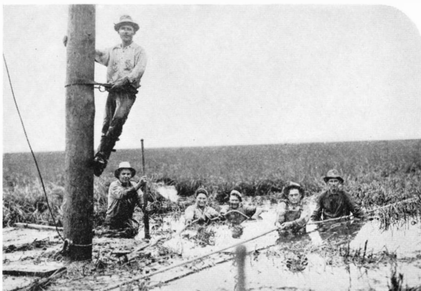
The difficulties faced by these linemen, who are shown stringing power and telephone wires, exemplify those faced in the entire job of building the plant
