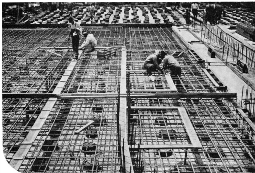
The mats on which piers are constructed to support building floors are built of concrete heavily reinforced with steel directly on top of the sawed off piles
