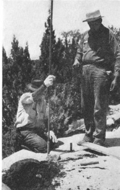
"X" marks the spot for the next pole. Whether there be mud or sand, or rock that must be blasted out, that spot is where the pole must go
