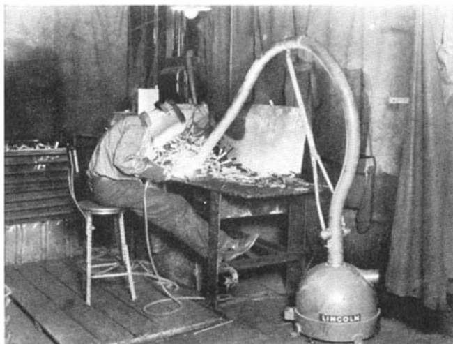
Air conditioning where it is most needed in a factory—at the source of air pollution. Carrying away welding fumes
