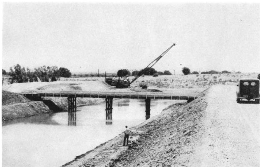
First part of the Central Valley Project to be constructed is this initial four-mile section of the great Contra Costa Canal, which will be 46 miles long
